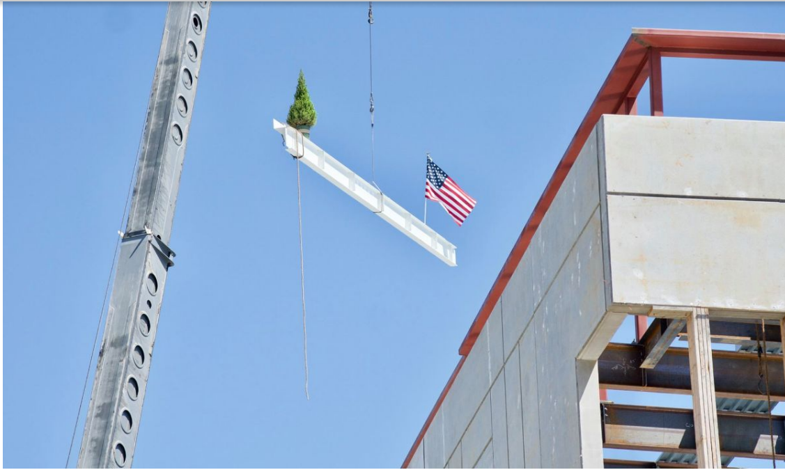
The Spruce tree on the Be Well OC beam is an old-time tradition that symbolizes good luck.
